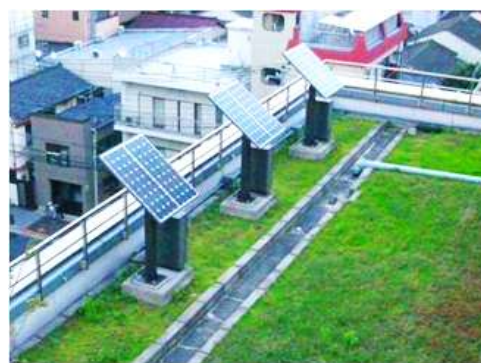
Olinas Tower (Solar power generation equipment)
