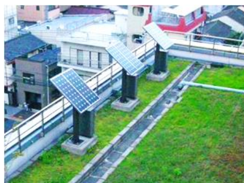
Olinas Tower (Solar power generation equipment)
