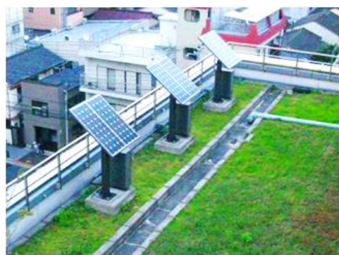
Olinas Tower (Solar power generation equipment)
