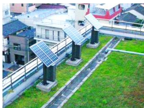
Olinas Tower (Solar power generation equipment)
