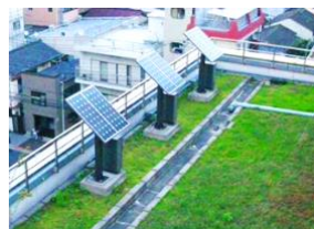
Olinas Tower (solar panel)
