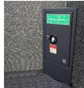
[Elevator emergency box]
