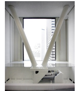
Newly installed seismic damper
