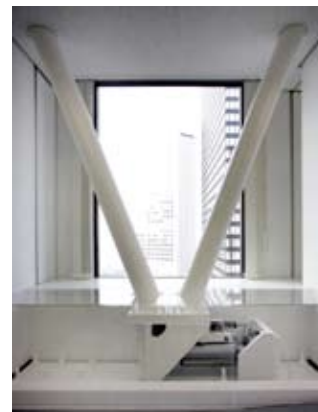
Newly installed seismic damper
